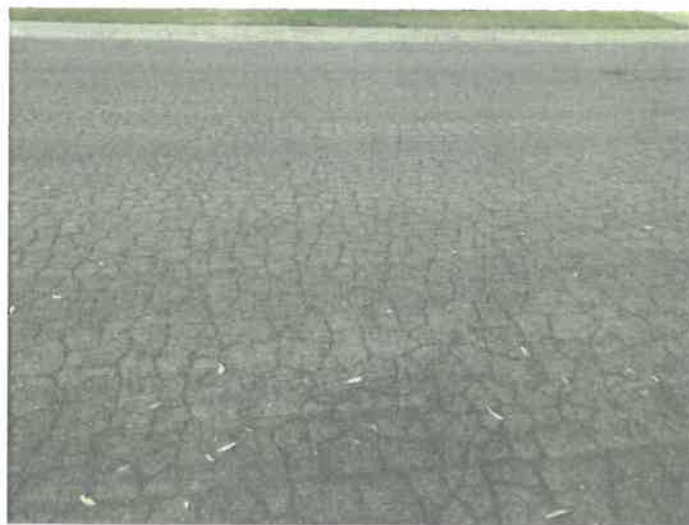
Example of: Medium severity alligator cracking - Harris St between 19 th St and Hall St (PCI 18)
