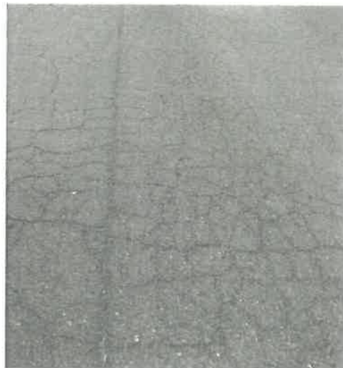
Example of: L+T cracking with Alligator cracking - Huston St near Johnson St (HUS_JOH_22: PCI 11)
