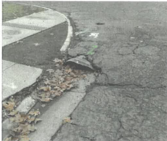
Example of: Raising pavement at the culvert at the intersection of I St and 12 th St (PCI 34)
