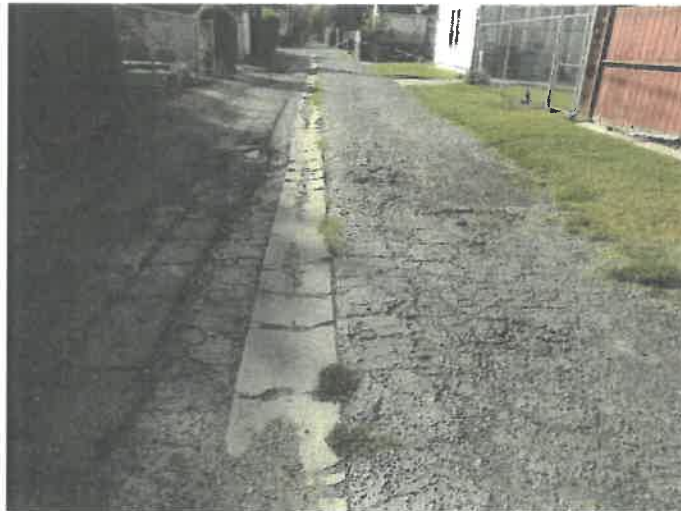
Example of: High severity raveling, weathering, depression, and pothole, along with medium severity L+T cracking, alligator cracking, and utility cuts - Pine St between 6 th St and 7 th St showing (PCI 7)
