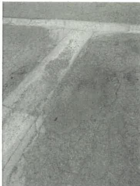
Example of: Pothole on Freeman St at the intersection with 13 th St (PCI 11)
