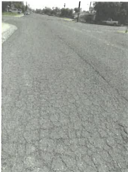
Example of: Combination of weathering and high severity alligator cracking E19th St at the intersection with Sampson St, showing (PCI 8)
