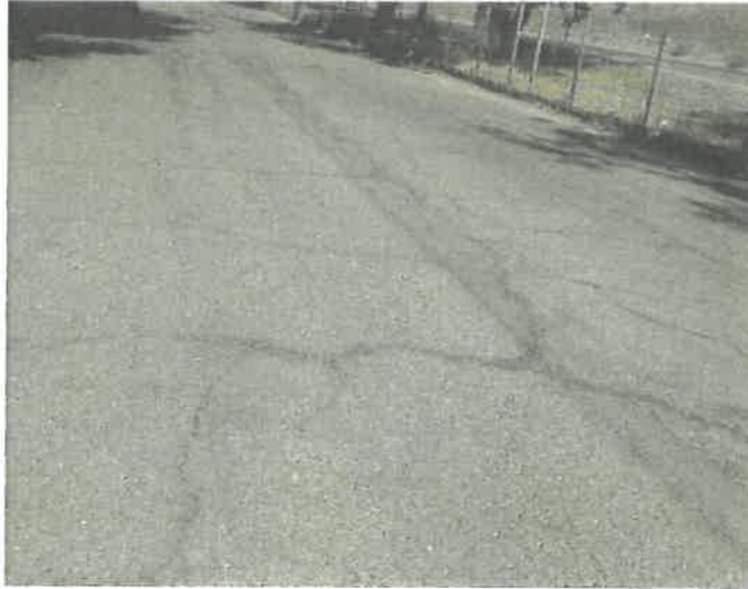
Example of: Block Cracking on Glen St between Rideout St and 17 th Street (PCI 20)
