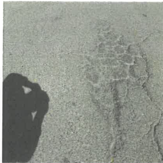
Example of: Medium severity localized alligator cracking - C St between 2 nd St and 3 rd St (PCI 26)
