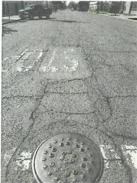
Example of: Failing utility trench patch – 12 th near E St (12TH_E_F: PCI 53)
