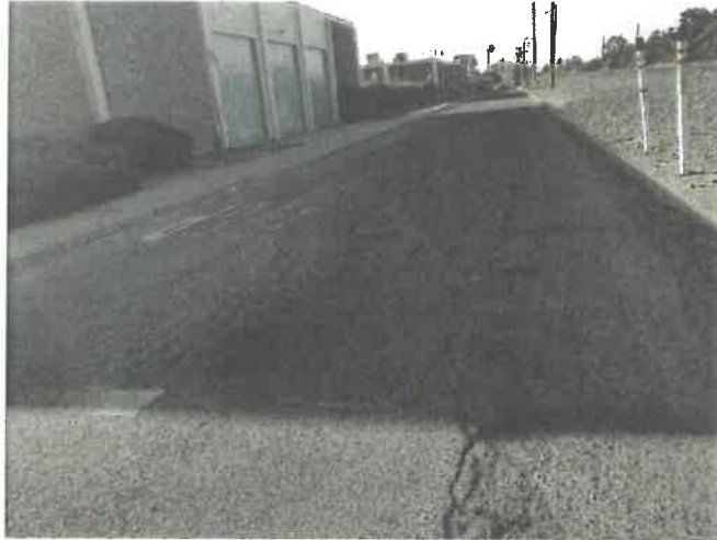
Example of: Potholes, weathering, raveling, cracking, alligator cracking - A_6_4 intersection at 6 th (PCI 7)
